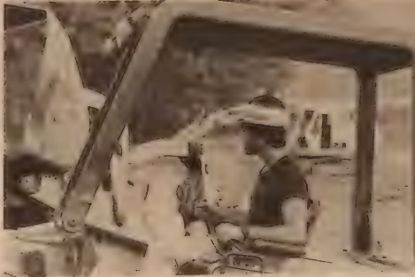
Edward J. Stellar, of Kulpmont excavating the land on a John Deere truck loader
